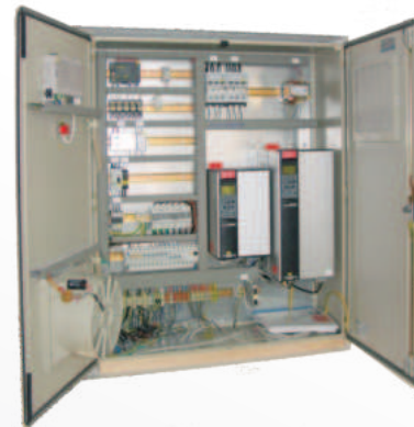
Switch board exhaust unit
