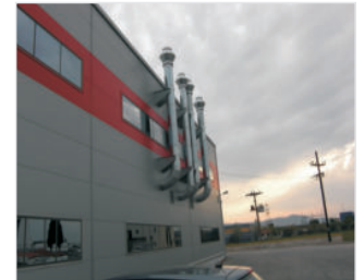
exhaust air with deflector hoods
