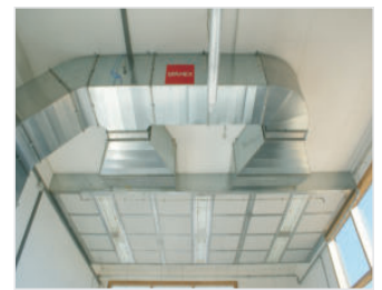
supply air ceiling with lighting
