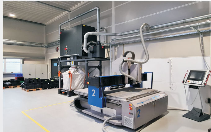
Central extraction system with supporting fan
