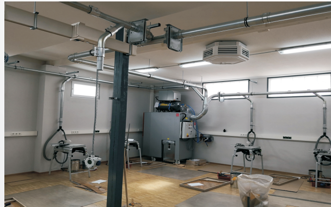
Extraction system in a training workshop
