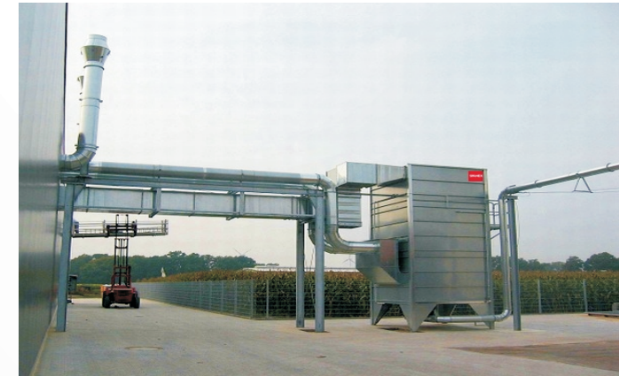
Image 2: Stationary filter system, air quantity capacity 40,000 m 3 /h
