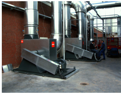
exhaust fans with sound insulation
